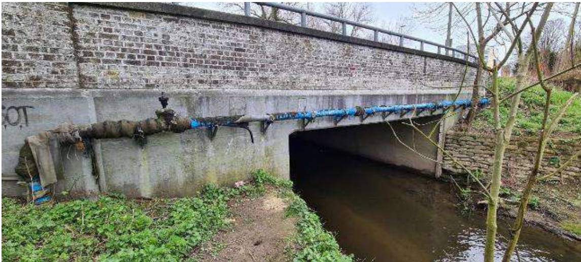
Figure 11: View of the A23 Brighton Road bridge over the River Mole from the North
